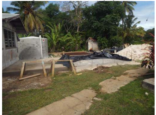
Foundation site for the Atiu coconut oil project (Photo provided by Techelle Punua)
