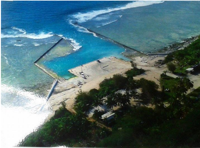
The revamped Mangaia harbour built to withstand more intense cyclone events presented by Paul Maaote (Photo by Paul Maaote)
