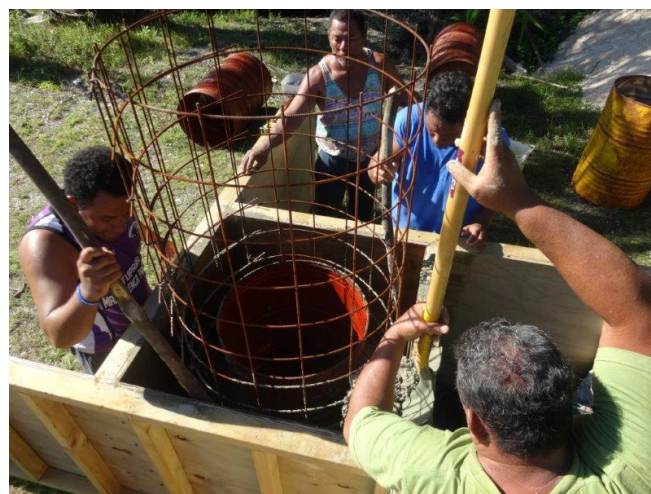
Community workers in Pukapuka preparing mold for culverts (Photo provided by Lucky Topetai)
