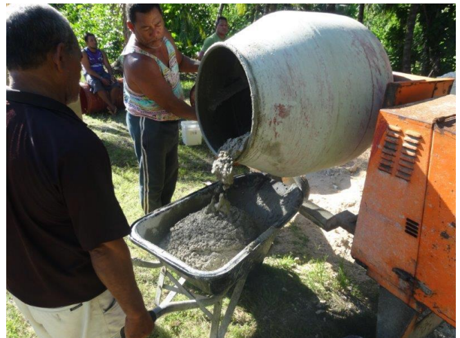
Men on Pukapuka churning cement to construct the moulds for the culverts to drain flood waters from the taro plantations 27 May 2016
